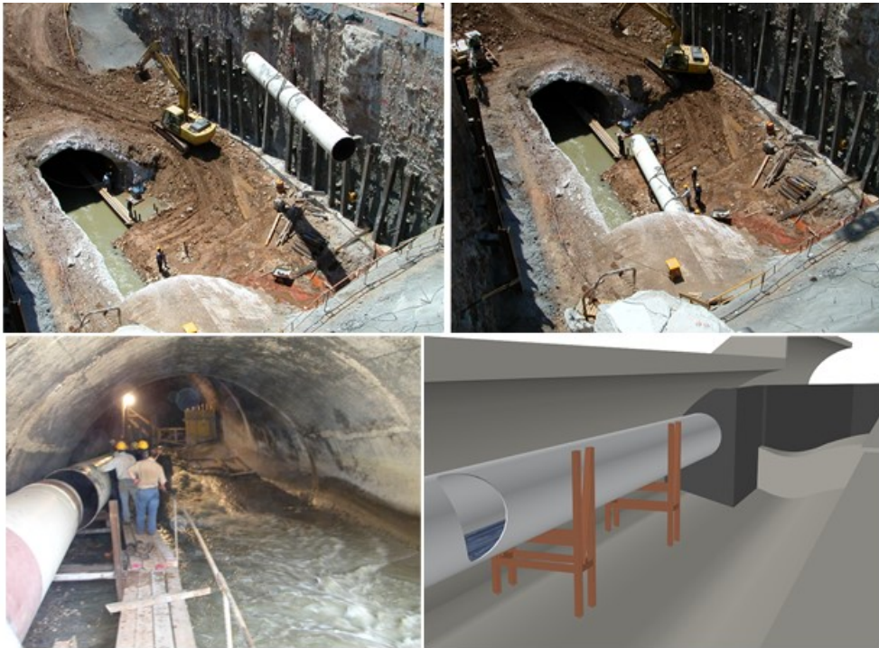
Images and schemes of the flow by-pass solution executed along the extent of the damages detected in the tunnel structure
