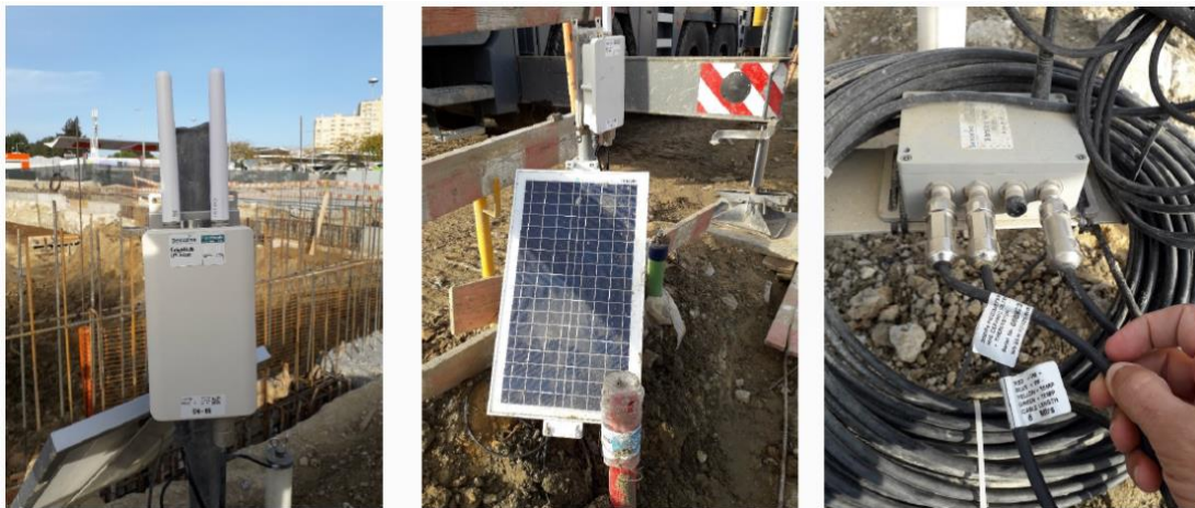
Figure 6 - Automated monitoring installed in plot 1
