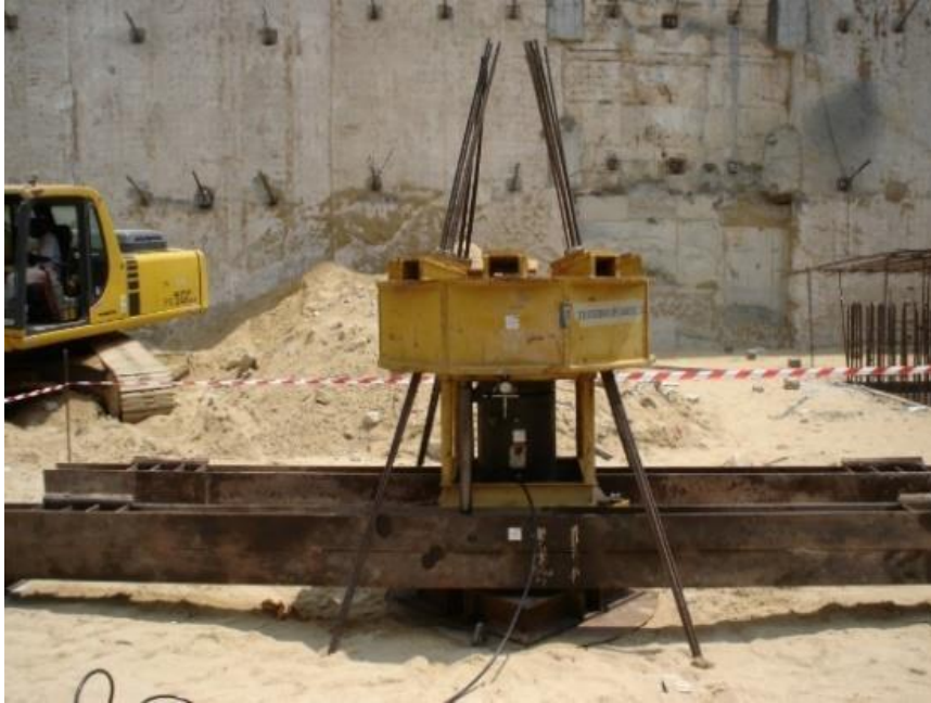
Load test with a circular \phi 1.5 m plate with loading imposed by prestressed ground anchors
