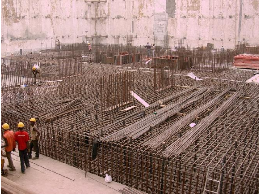
Slab reinforcement cage with incorporation of the steel CHS pipes through which the injection was executed
