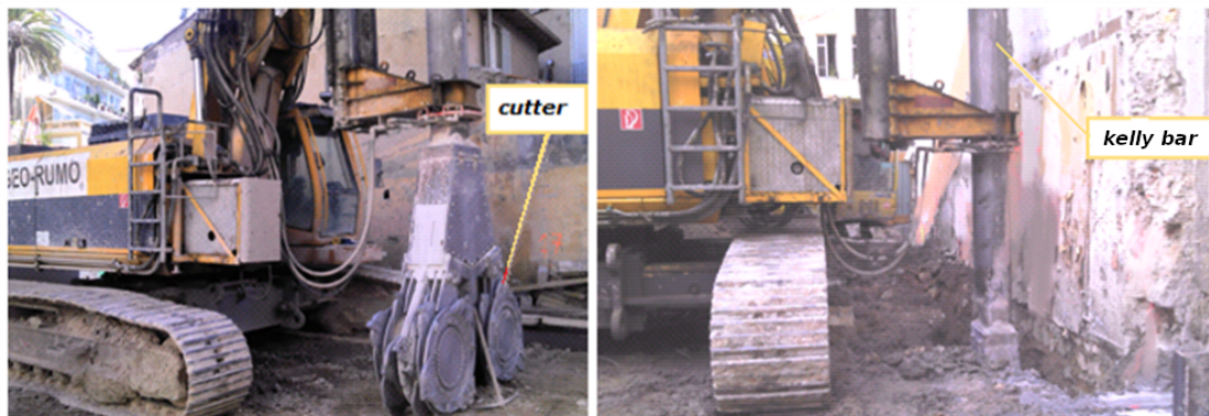
Equipment and cutting tool (left) and execution of the CSM panel (right)
