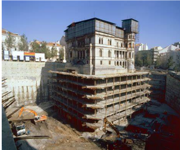
View of the Palace's support and shoring system in the final stage of excavation
