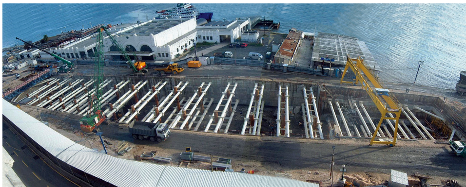
View of the curtain and shoring system from the Terreiro do Paço east tower
