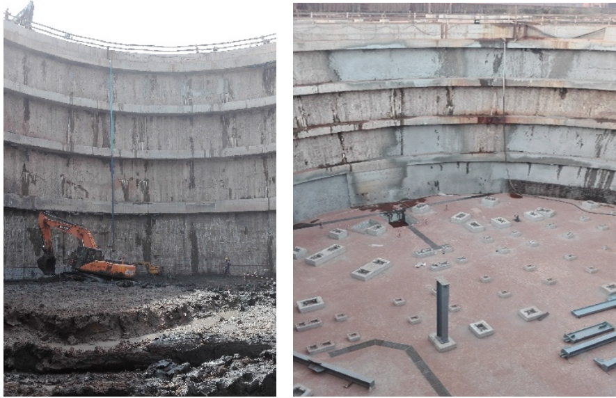
Diaphragm wall and retaining beams in the final excavation phase and after completion of the bottom slab
