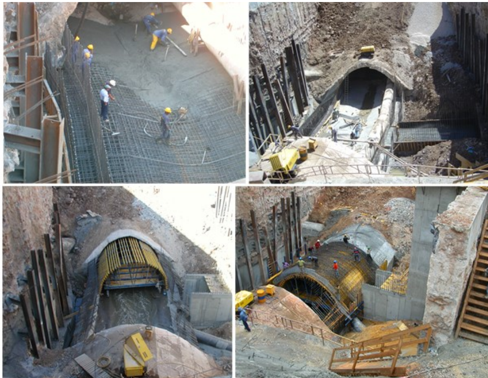
Images showing the main sequential phasing used for the reconstruction of the tunnel's structure
