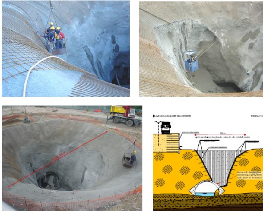
Images and schematics of the solution for the provisional stabilisation of the crater created by the rupture of the tunnel
