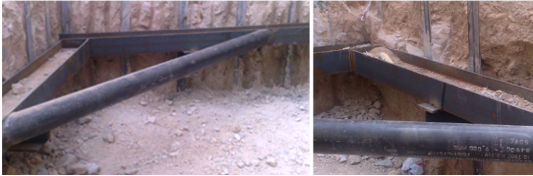
Detail of the steel distribution beam directly connected to the vertical profiles of the retaining wall
