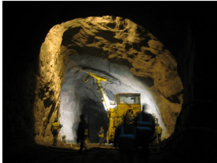
Beginning of cavern excavation by the longitudinal gallery on the water intake side (turbination)
