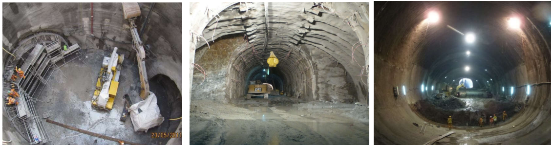
Access shaft, top heading and final section construction of the Place des Martyrs Station
