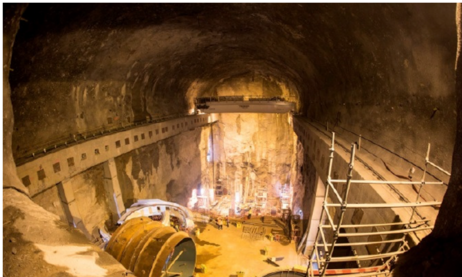
Excavation of the power plant. In the foreground, the assembly hall. In the background, the area of the pumping unit
