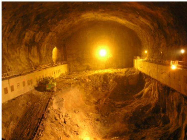
Excavation of the entire dome and execution of the anchored beams of the overhead crane. Ramp and excavation of the lower level
